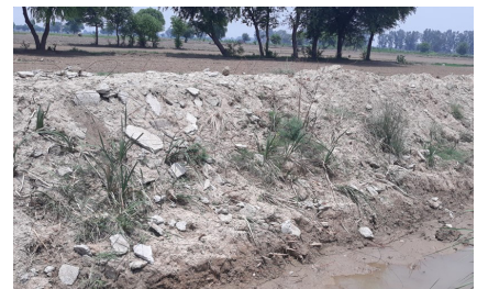
Failure of the concrete in drain canal
