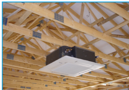
Air conditioning units
