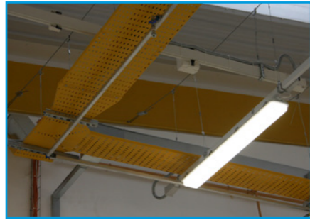
Busbar and Lighting
