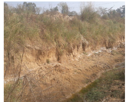
Erosion in the channel before Gripple install
