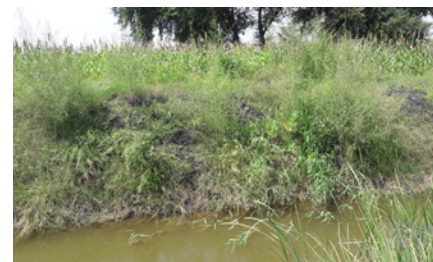
80 days after installation
