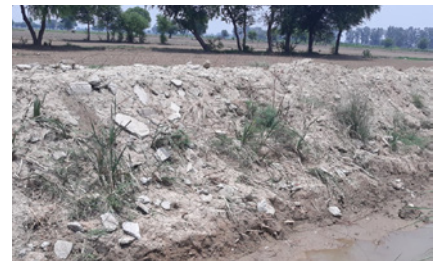
Failure of the concrete in drain canal
