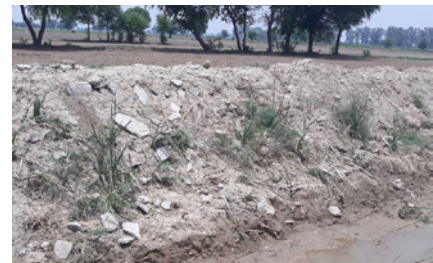
Failure of the concrete in drain canal
