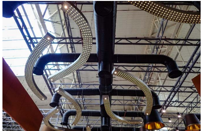
Food court HVAC ducting
