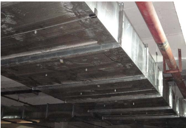
Carpark HVAC ducting
