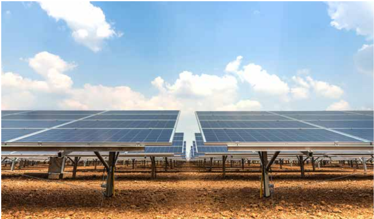
Solar Bracing and Anchoring
